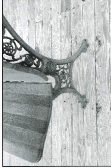
Evidence of the original desk benches being fastened to the floor was found under the top layer of flooring.
